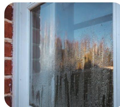
Misted Units Replaced
