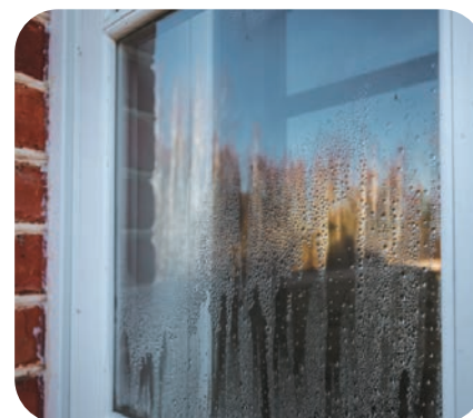
Misted Units Replaced
